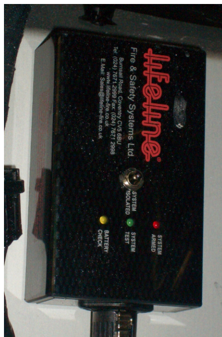
Extinguisher Control Box
